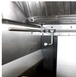
Flushing nozzles system
