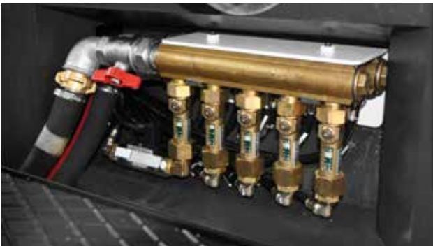
Five separate cooling circuits for the motors of the drives in the X, Y, Z, B/C axes, and the spindle motor.
