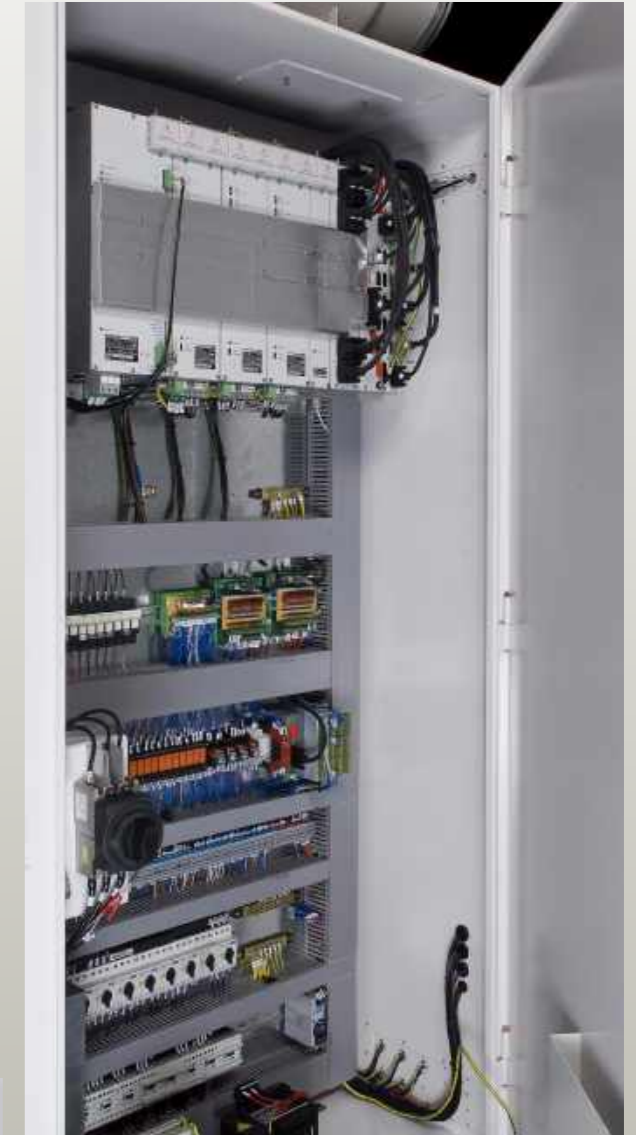
Electric System For Easy Maintenance
